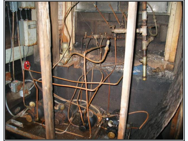
Residual Tank Piping
