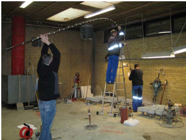
Indoor heater installation
