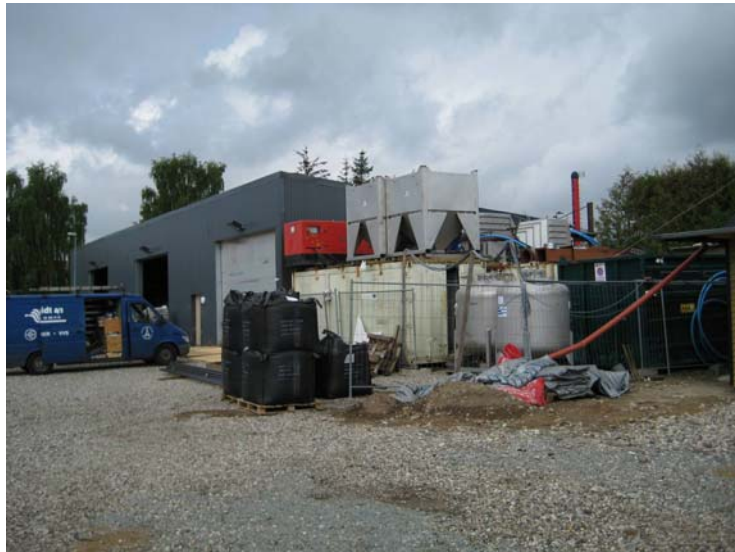
Treatment system in two levels due to limited space at site
