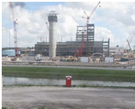
Palm Beach County Waste-to-Energy Project, April 19, 2013
