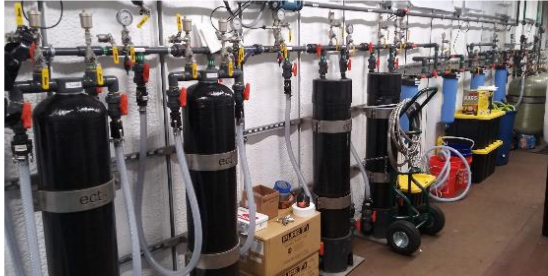
Ion Exchange Resin Vessels
