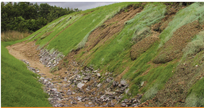
Slope Failure and Erosion
