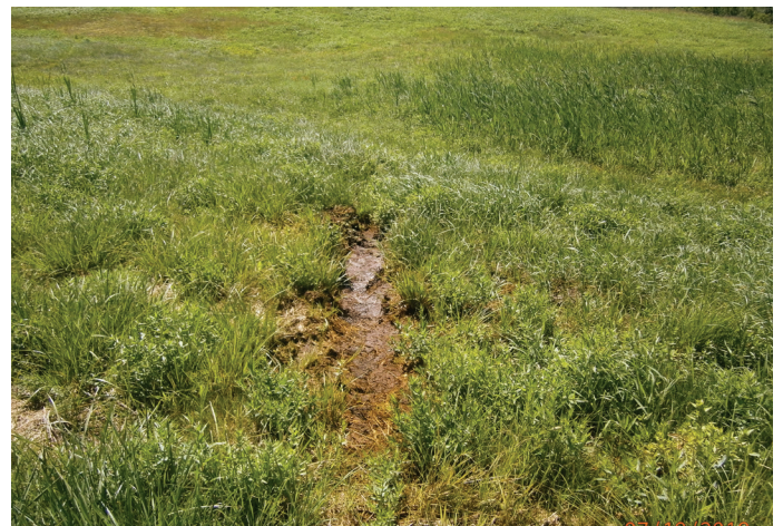
Leachate Seep on Landfill Side Slope
