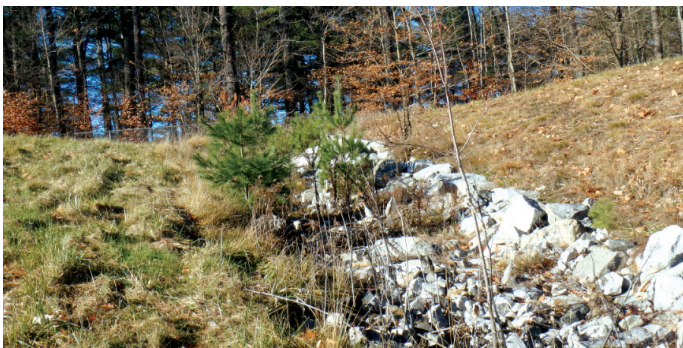
Woody Growth and Blocked Drainage Swale
