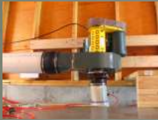
1) Turn on aeration blower
